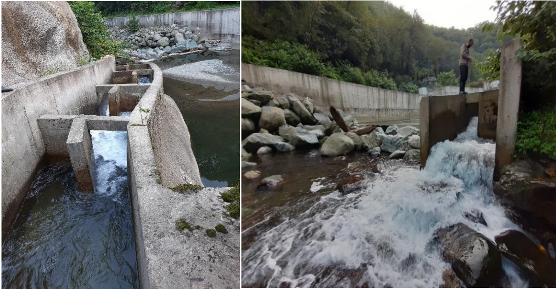
Figures 22. Fish passage (vertical slot fish ladder) on Kintrishi hydropower station dam.
